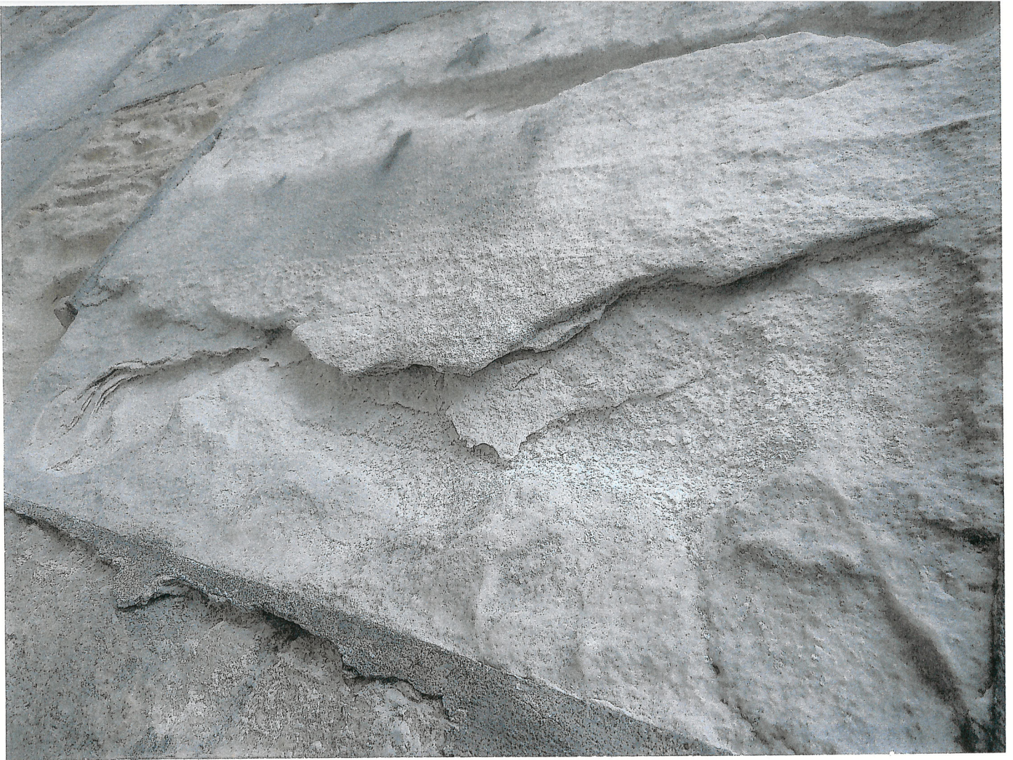
LAMINAR DETERIORATION OF MAGNESIAN LIMESTONE, YORK MINSTER, UK
