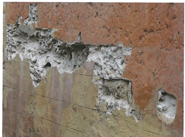
Two examples of the decay caused by impermeable cement mortar, which forces the limestone walls to dry through the stones. Salts accumulate in the stones which erode away, leaving the mortar standing proud. It's much cheaper and easier to replace mortar (repointing) than it is to replace stone.
