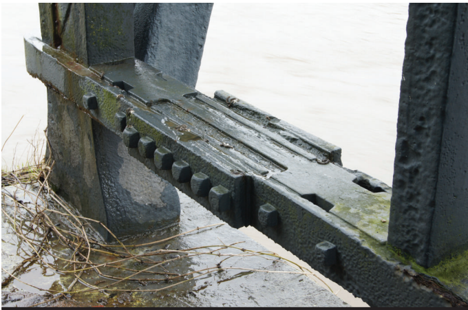
Figure 5 Iron Bridge, Shropshire. Intervention from 1902, providing greater integrity by tying together lower ends of five arches. In cast iron and mild steel, representing best practice at time
