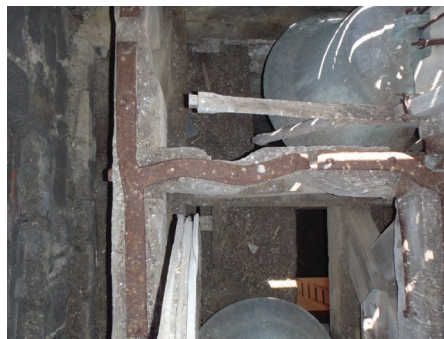
Figure 4 Wrought iron strap within 15th century church tower
