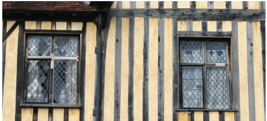
Figure 1 Timber window repairs at Ightham Mote demonstrate decision-making based on retention of original fabric
